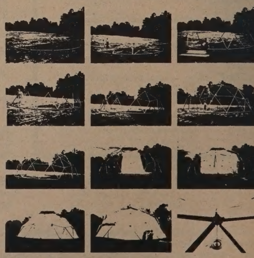
Fig. No. 101. Assembly sequence 55' diameter strut and membrane 1V Alternate dome. Note expansion sectors and pull-chain adjustment at spire casting.
